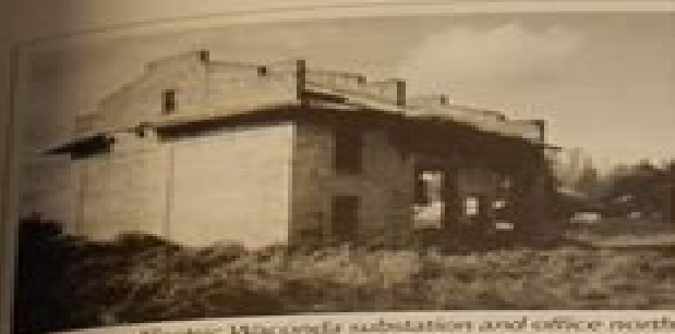
The Oregon Electric Waconda substation and office north of Salem, has thus far withstood more than 75 years of neglect. It served the dual purpose of housing both the transformers and the station itself. COURTESY BOBERT M. OWENS.
